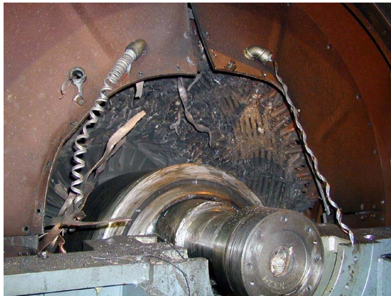
Figure 7 – Steam Turbine Overspeed Resulting in Generator Rotor Imbedded in Stator
