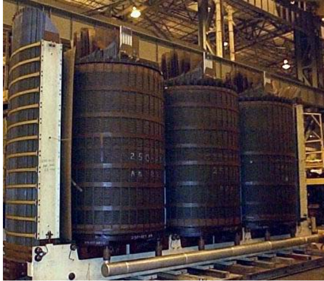
Figure 2 – Overheated 100 MVA Transformer
