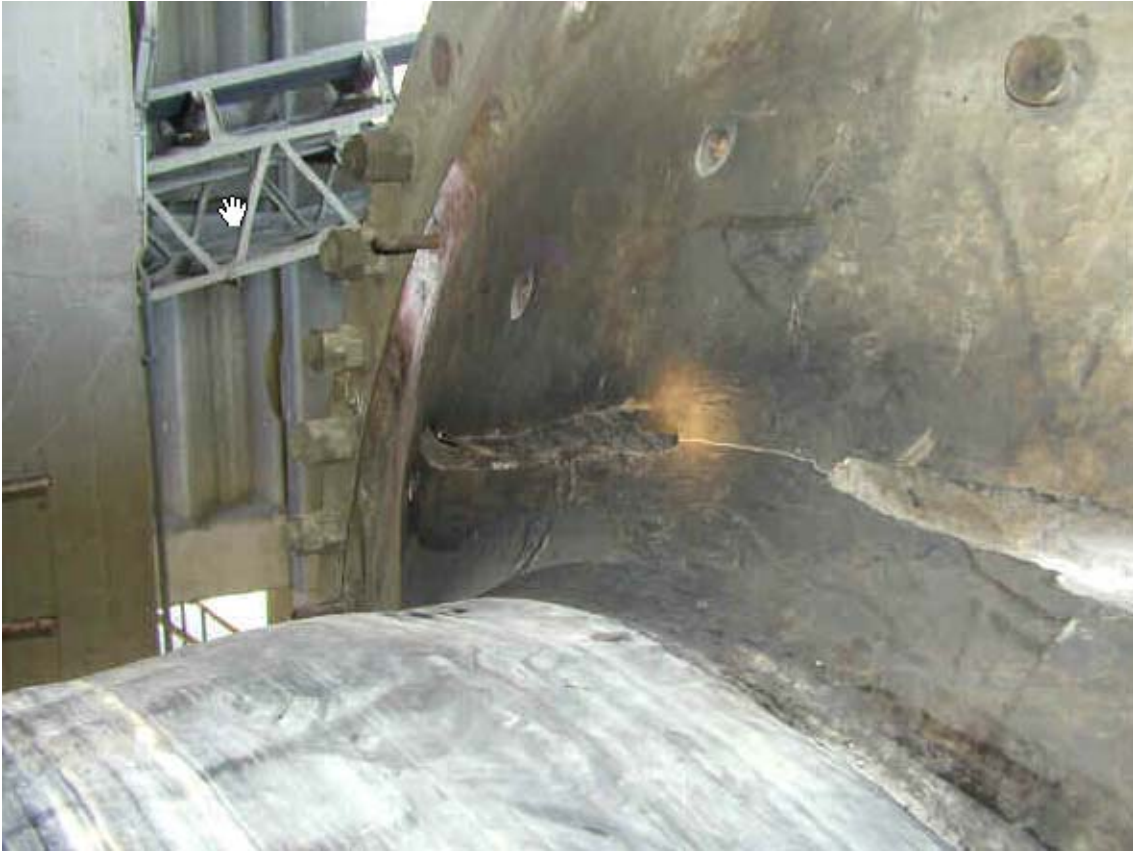
Figure 3: Outlet head; cracks are being repaired
