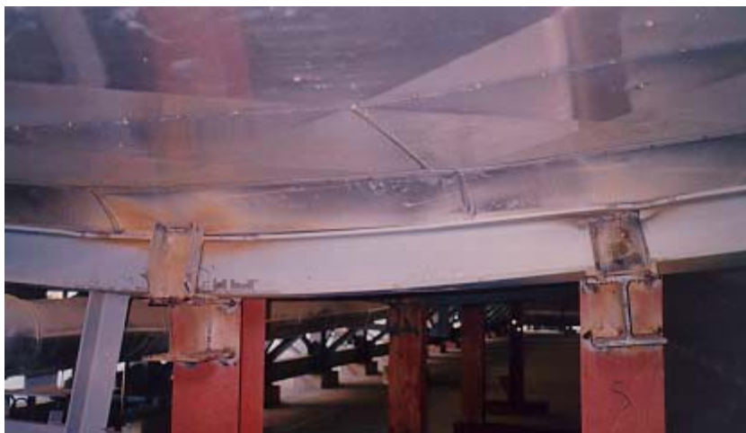
Deformation of H-beams and fractured welds
