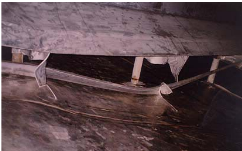
Deformation of separation wall and fractured seams
