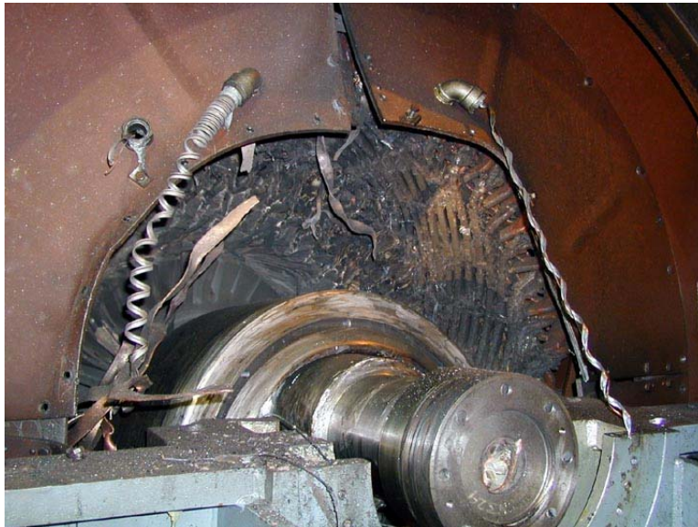
Figure 5 – Steam Turbine Overspeed Resulting in Generator Rotor Imbedded in Stator
