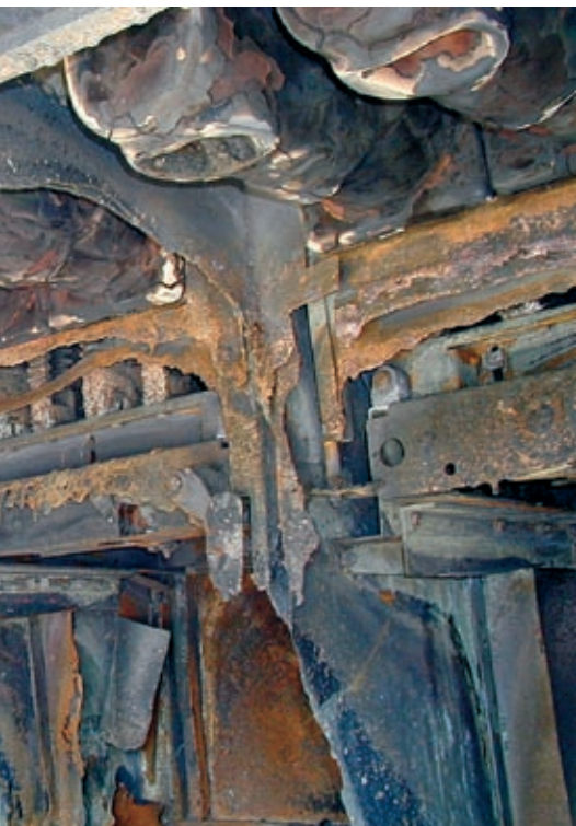
Picture 2. The temperatures created in an electric arc are extremely high (3 000 °C) and can evaporate e.g. metal parts which as the result of the created heat ignite combustible materials.
