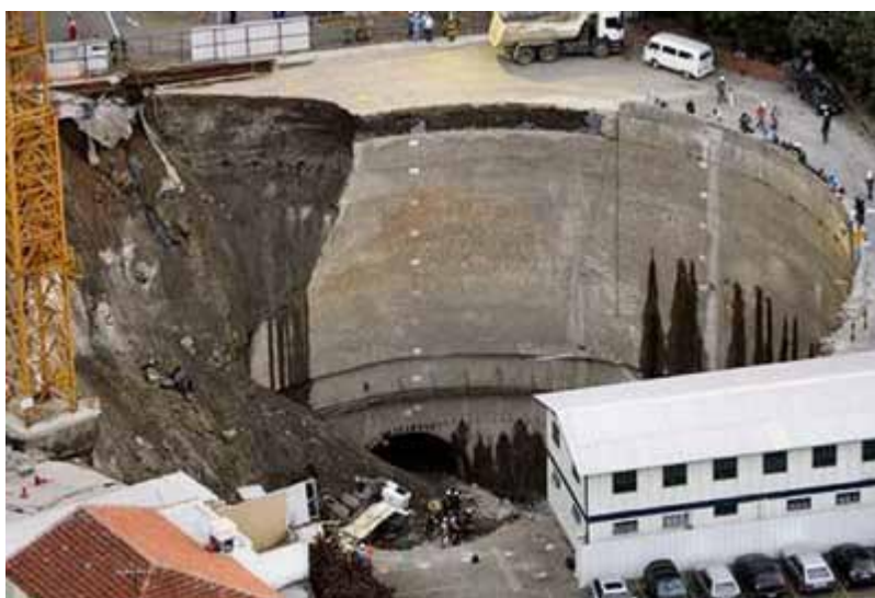
Figure 5. The Capri shaft after collapse, São Paulo Metro, 2007.
