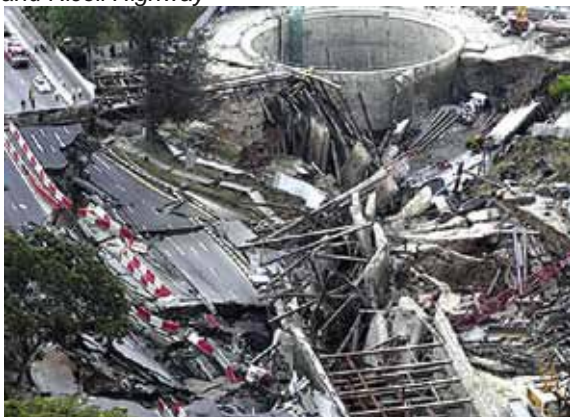
Figure 7. Failed Cut & Cover tunnel excavation and Nicoll Highway
