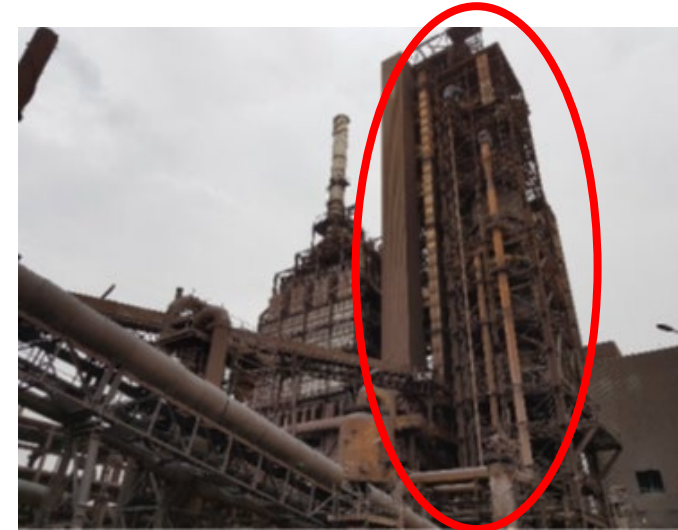
Process Gas Heater (left) DR Reactor (right) Courtesy of Emirates Steel (ES) Abu Dhabi UAE
