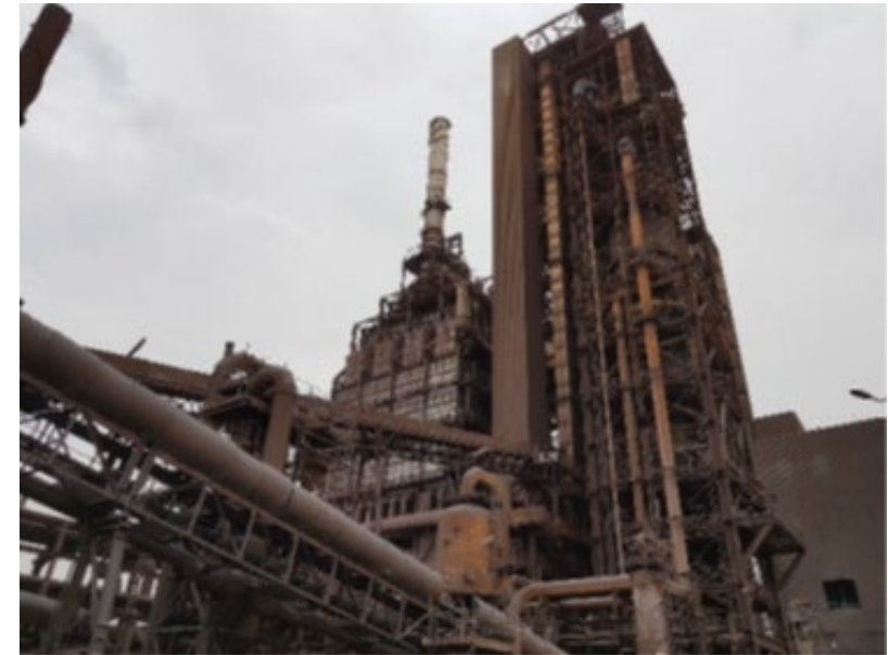
Process Gas Heater (left) DR Reactor (right) Courtesy of Emirates Steel (ES) Abu Dhabi UAE
