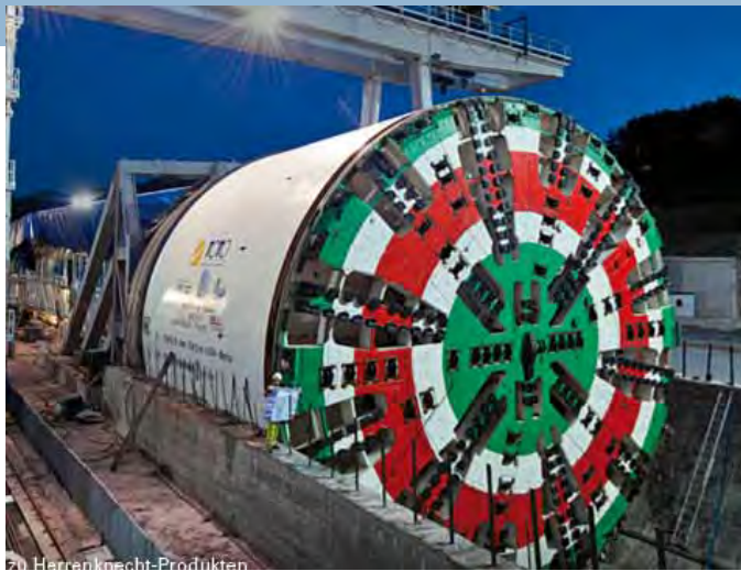
HERRENKNECHT MIXSHIELDS FOR LARGE DIAMETERS AND DIFFICULT GEOLOGIES.
