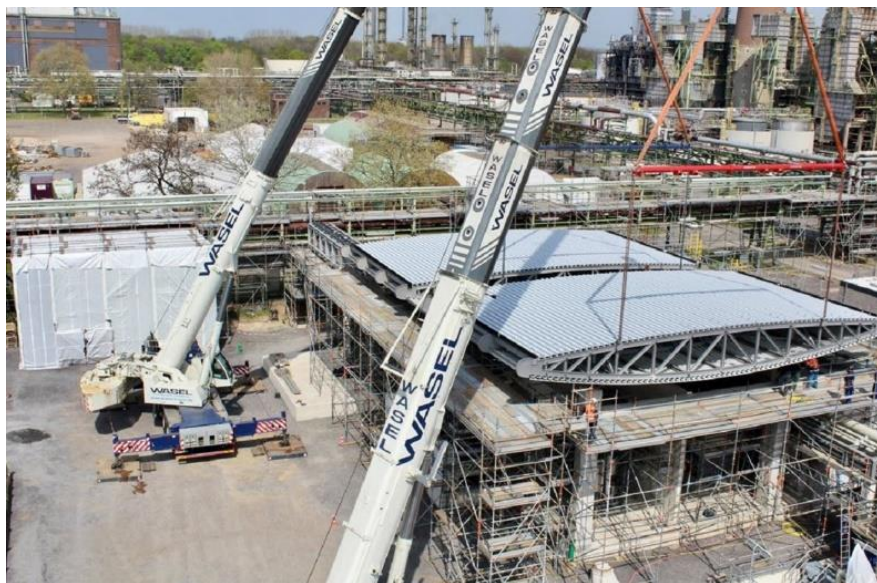
Hydrogen production building at the Shell refinery in Wesseling, Germany. Source: Shell Deutschland Oil
