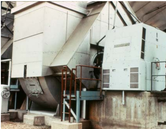
Figure 10 FD Fan Hartford Steam Boiler
