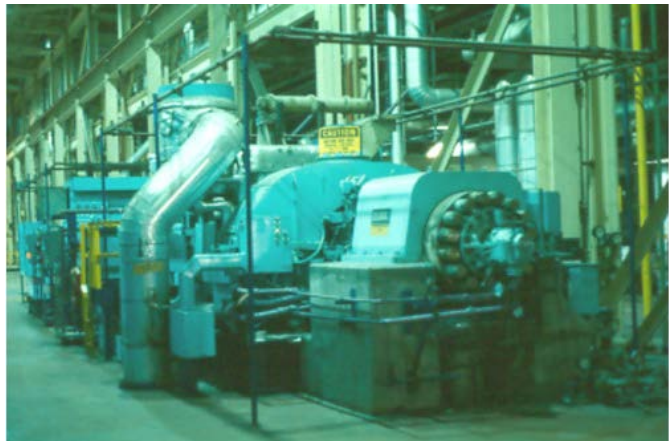
Figure 11 – Steam driven boiler feed pump Hartford Steam Boiler
