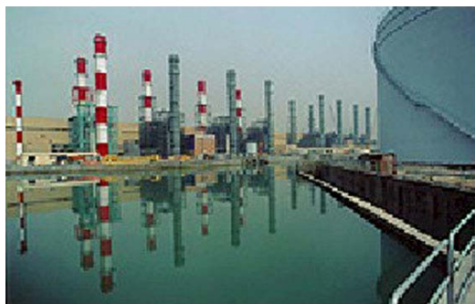
Photograph 2: The 2,000MW Seoinchon combined-cycle plant is located on the island of Ildo, 40 miles SE of Seoul, Korea.
