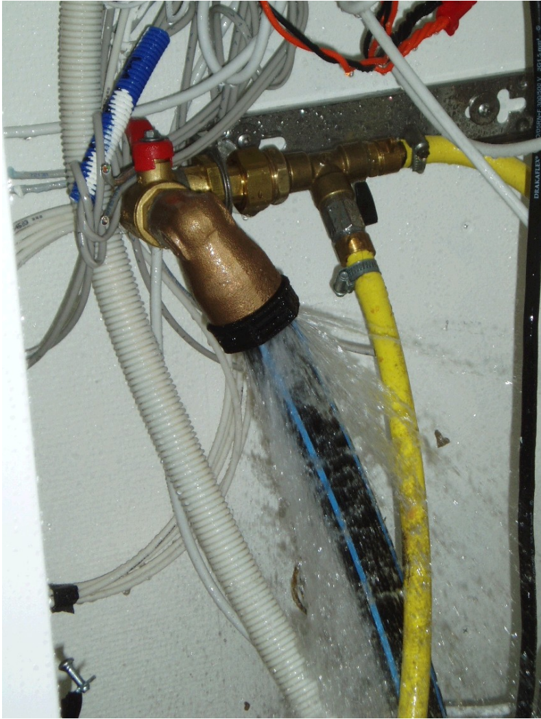
The cause of loss, a not correctly tightened coupling came loose due to faulty workmanship.
