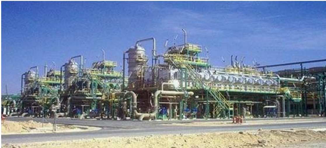
View of a MSF plant
