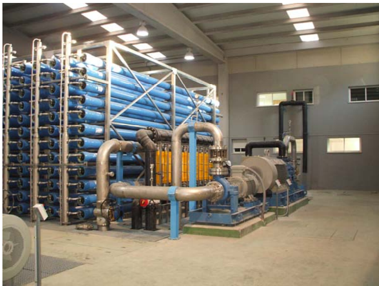
Typical membrane frame with high pressure pumps
