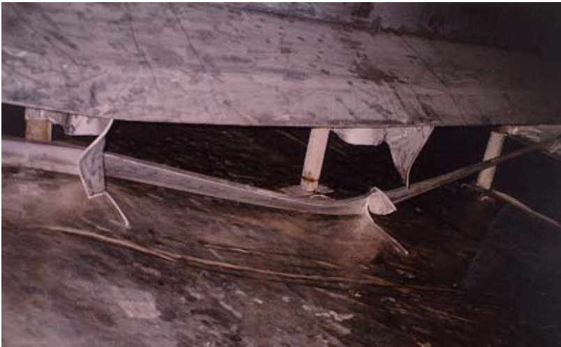
Deformation of separation wall and fractured seams
