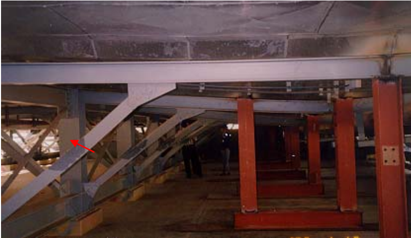
Deformation of supports, in evidence of protective coat chipped off
