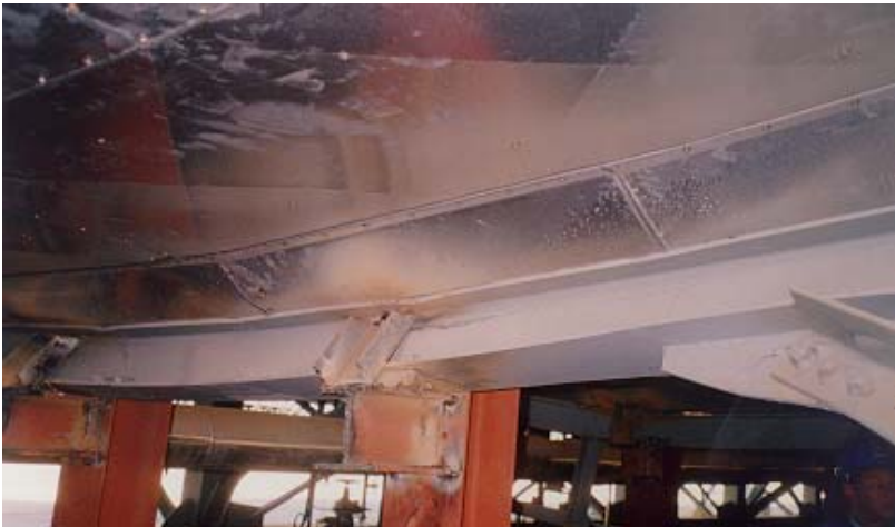
Deformation of H-Beams and fractured welds
