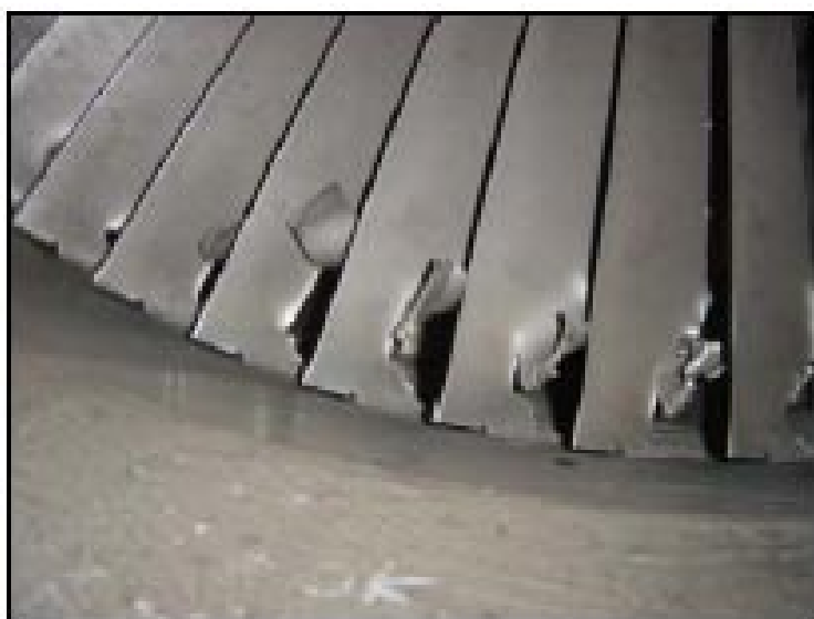
Figure 7: Endoscopy of a compressor section in a gas turbine with foreign object damages (FOD)
