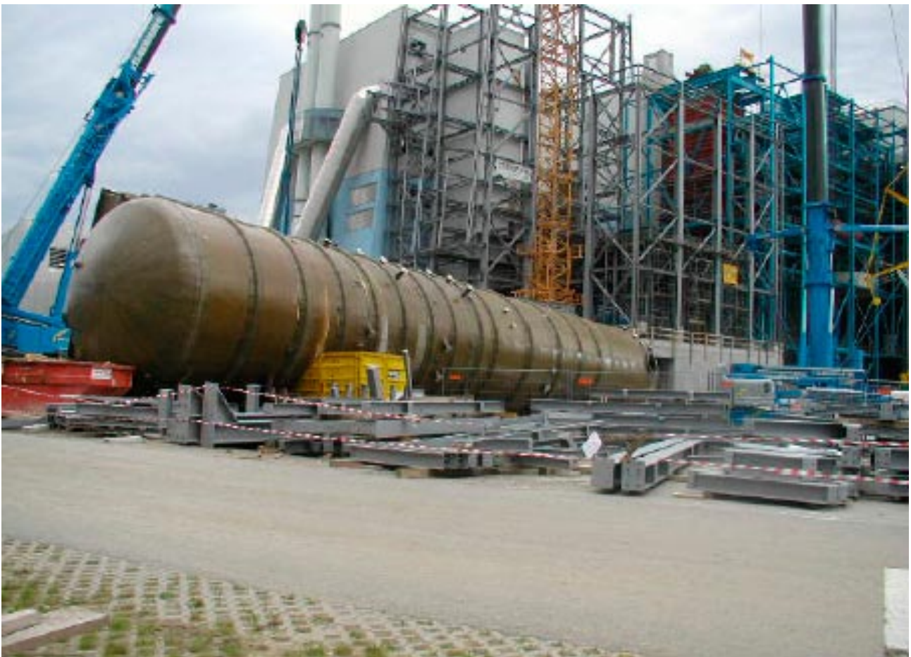
Scrubber vessel with the two cranes after the occurrence
