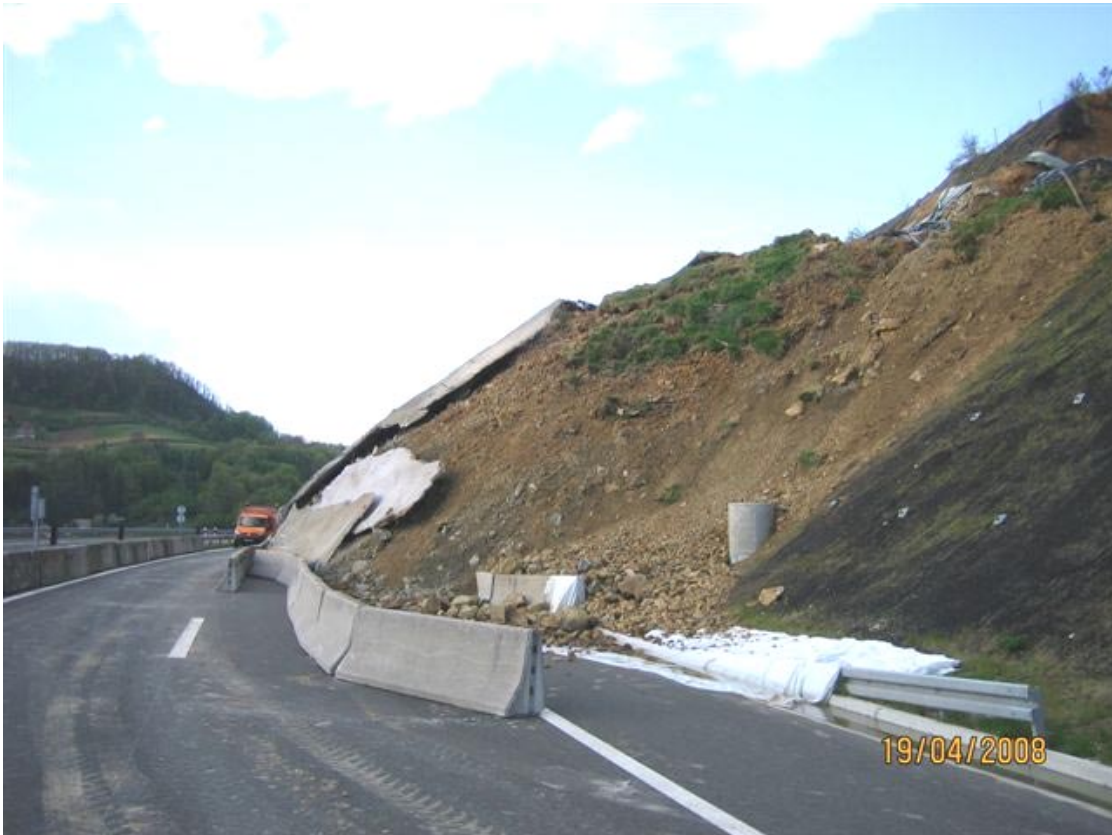
Situation shortly after the landslide occurred
