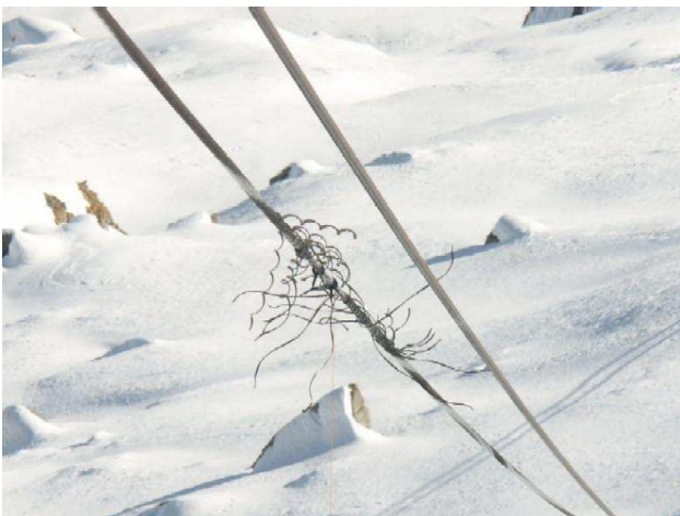
Damage on the track cable wire
