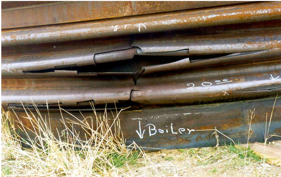
Figure 15: Cracked compensator of gas turbine exhaust
