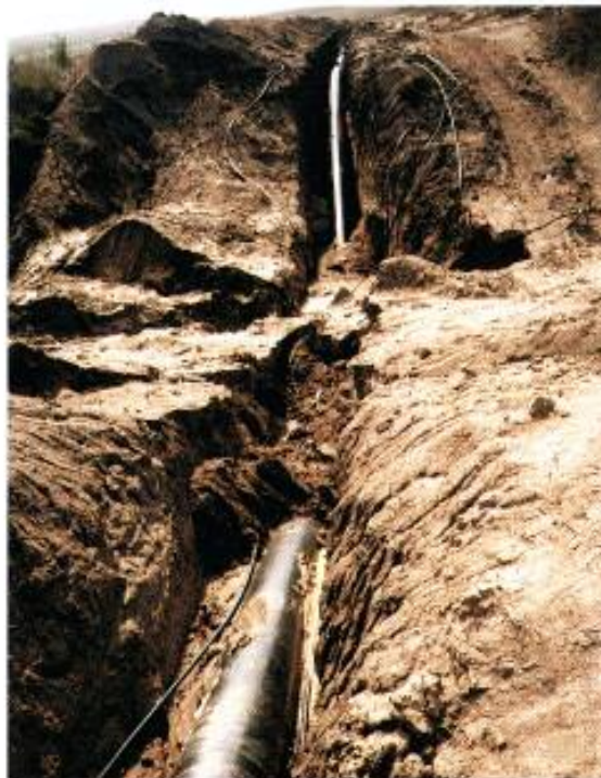
Slide No. 207 Eroded and collapsed trench slopes
