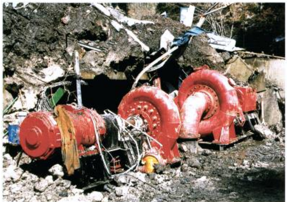
Slide No. 142 A close-up of the above site gives a better view of damage to the installations.
