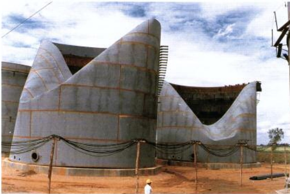
Two damaged items out of 14 fuel tanks
