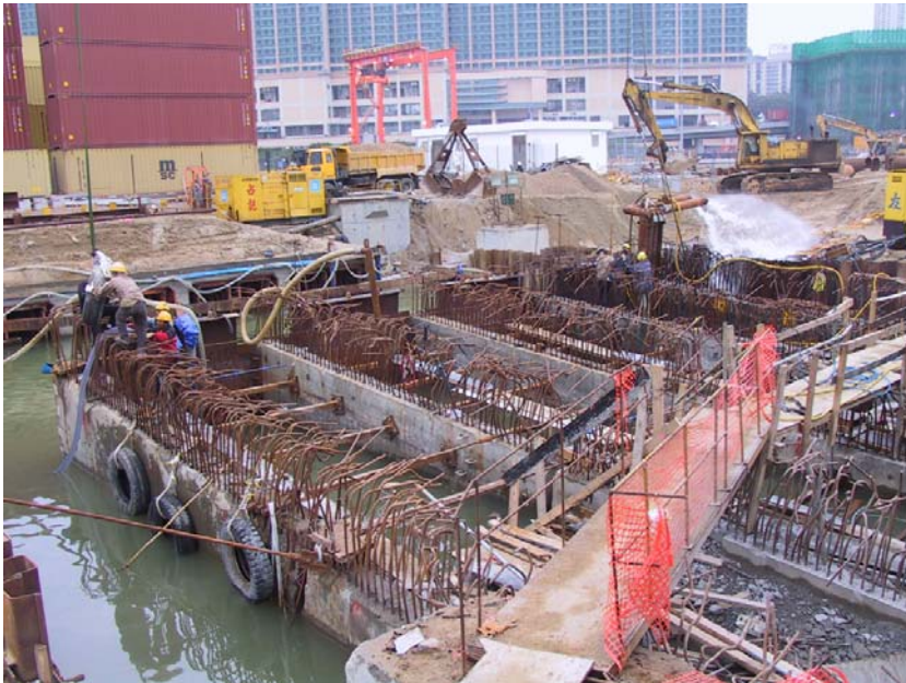
Tilted outlet structure
