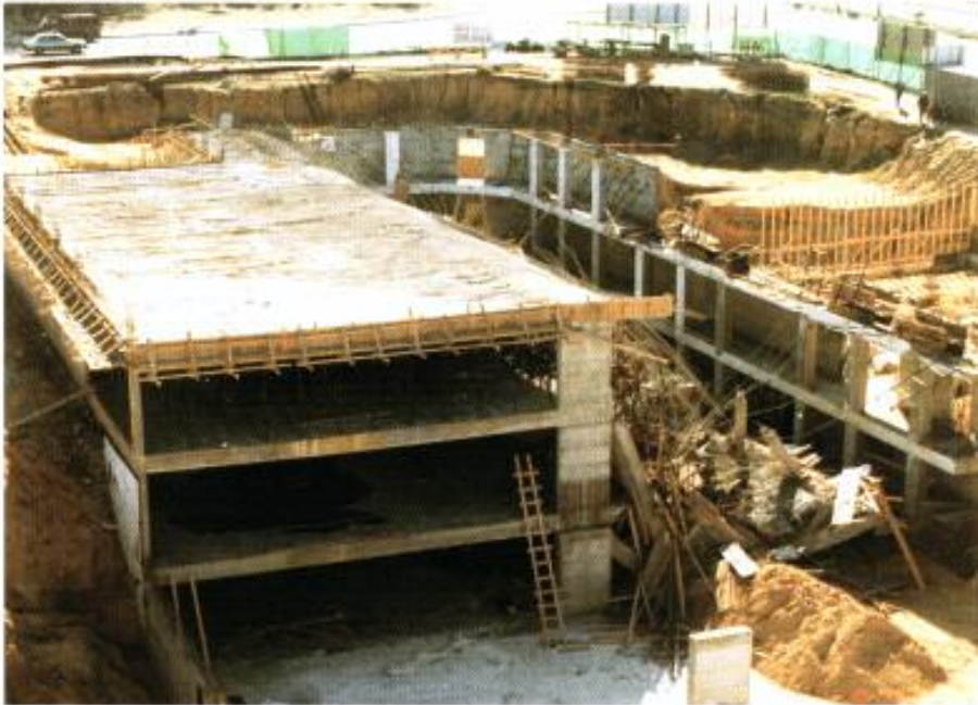
Slide No 108 Collapsed middle section of underground car park
