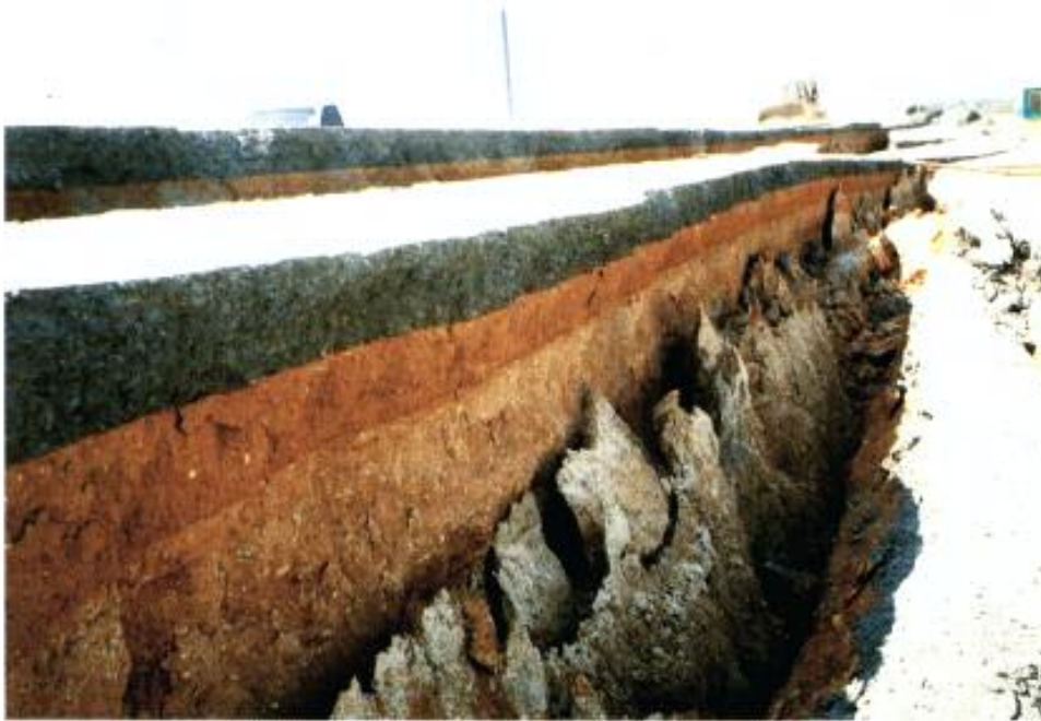
Backfilled embankment after soil collapse. Destroyed asphaltic layer fell into opening gaps.
