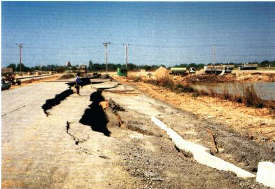
Subsided road embankment in close vicinity of a pond
