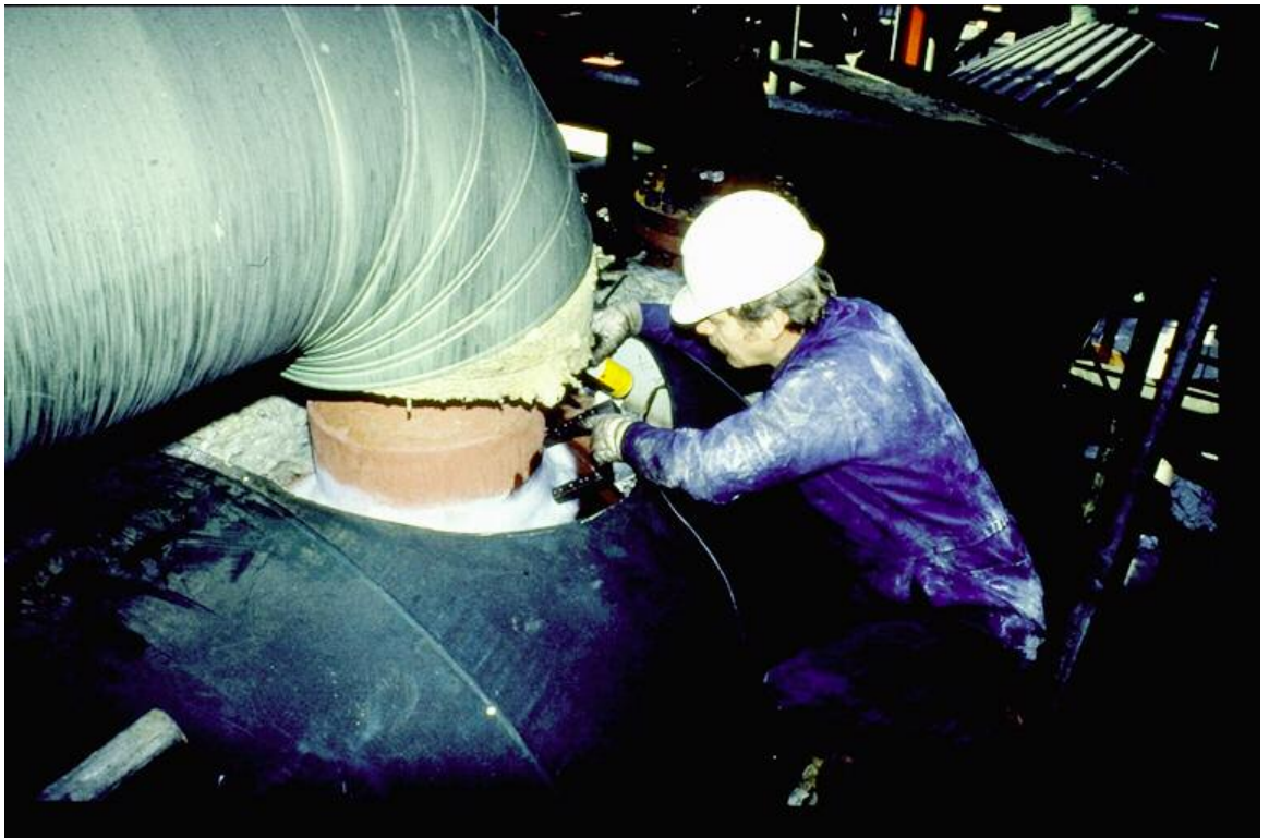
Figure 9. Magnetic particle testing of a steam pipe in a power plant using a yoke and white contrast paint before applying the black suspension from a spray can
