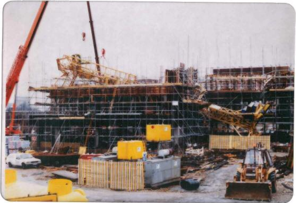
Figure 3. A broken tower crane. Failure caused by internal corrosion
