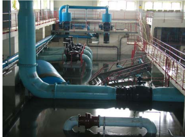
Fig. 11: Power plant after Flood
