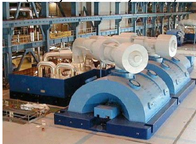
Figure 4 – 1,050 MW Cross Compound Steam Turbine Generator (Courtesy Mitsubishi Heavy Industries)
