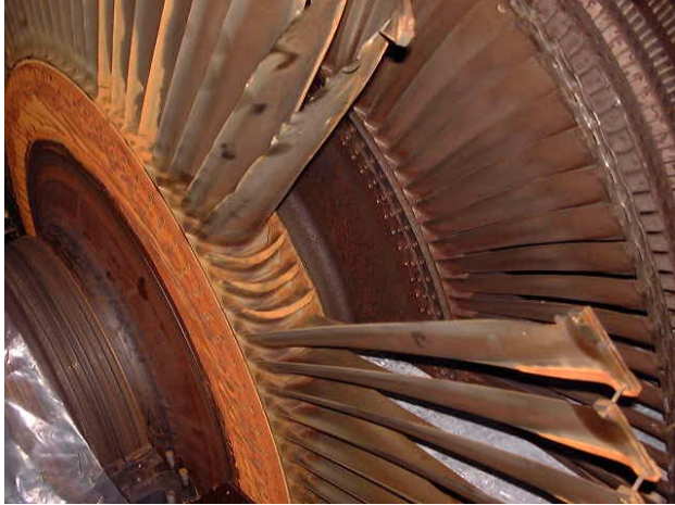
Fatigue Failure Compounded by Condenser Extraction Line Backflow
