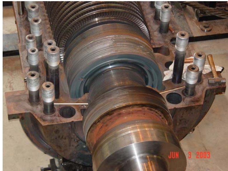
Rotor/Seals Welded to Inner Shell from Rub
