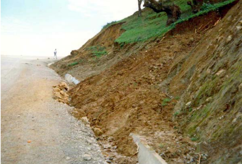
Photo No. 2: Landslide occurred at locations with shallow cut angles.
