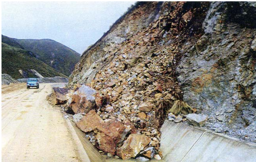
Photo No. 3: Damaged concrete canal by fallen rock. Slope angle too steep, insufficient drainage.
