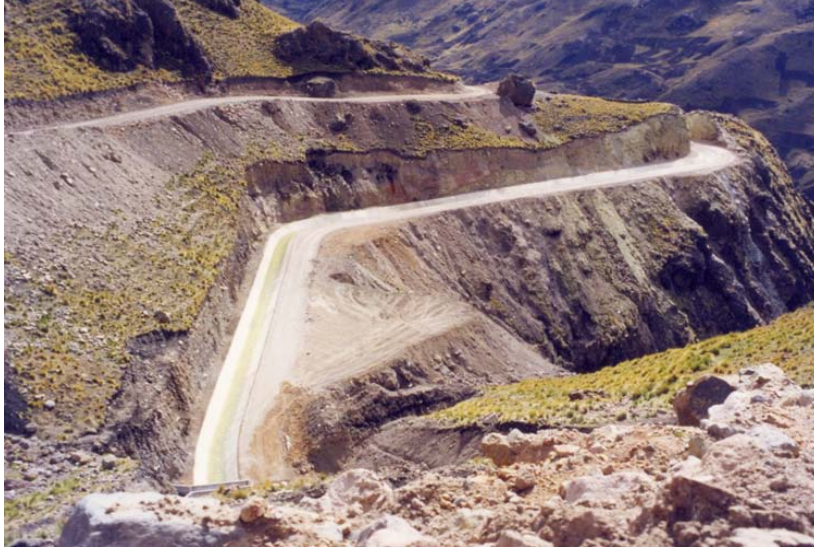
Photo No.1: Construction of road and canal of 40km length on slope of the Peruvian Andes, at heights reaching 5.000m asl. The project is for collection and routing of rain water for irrigation of agricultural land at lower levels.
