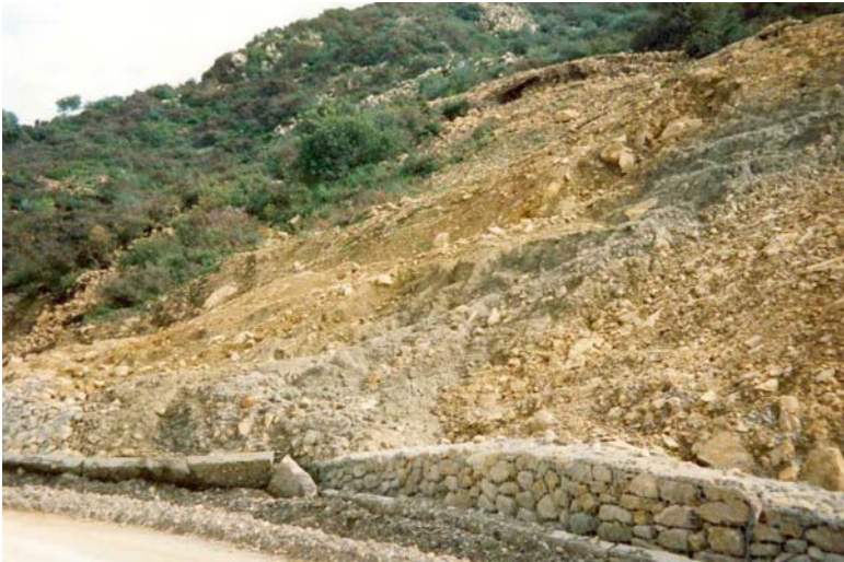
Photo No. 3: Benched slopes and gabions damaged by slides
