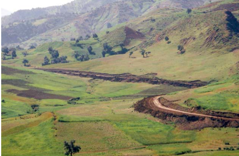
Photo No.1: Construction of 60km new road network as due to the dam construction existing roads below 168m asl located within water reservoir of the dam. Slides due to inadequate drainage above slopes.
