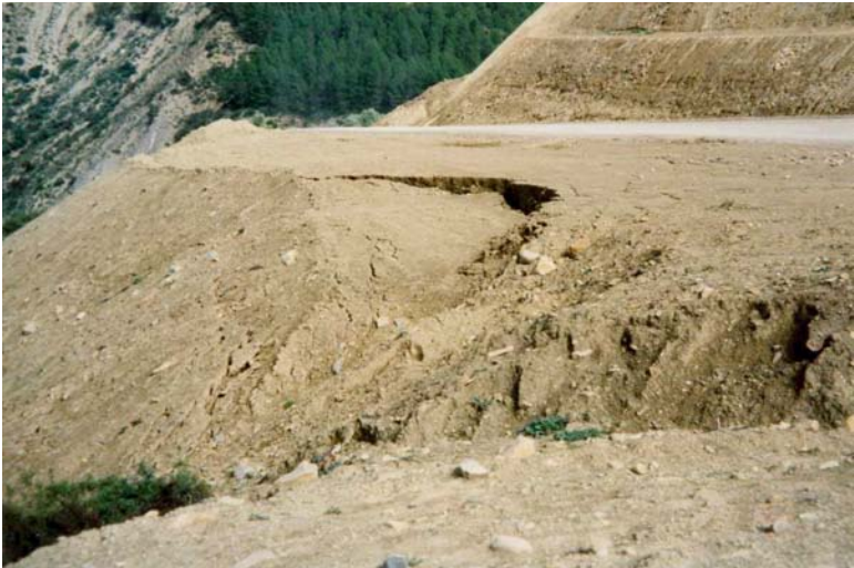
Photo No. 4: Damage to filled road structure after heavy rainfall.
