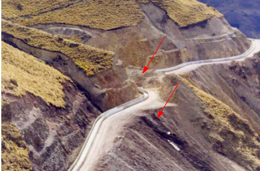
Photo No. 2: Completed road and canal section after landslide.
