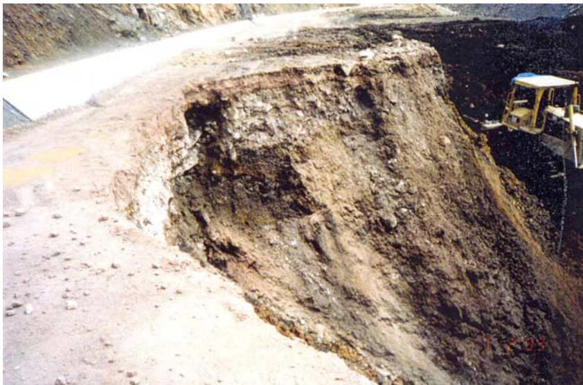
Photo No. 4: Landslide road structure slope stability not adequately secured.
