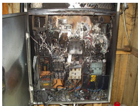
Short circuit in a power panel. Root cause was lightening.
