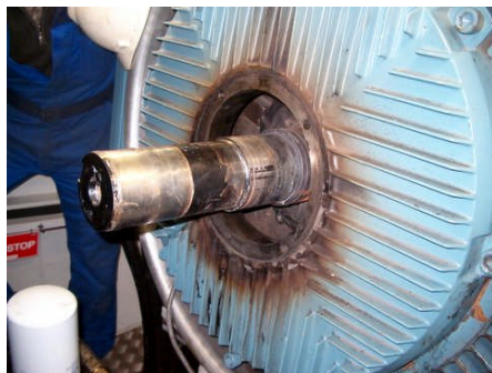
Hot bearing from a 1 MW generator. Root cause could among others be lack of grease, unsuitable grease or loos connection between bearing and shaft.
