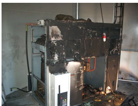
Short circuit in a power panel. Root cause was a bad connection on a high power cable.
