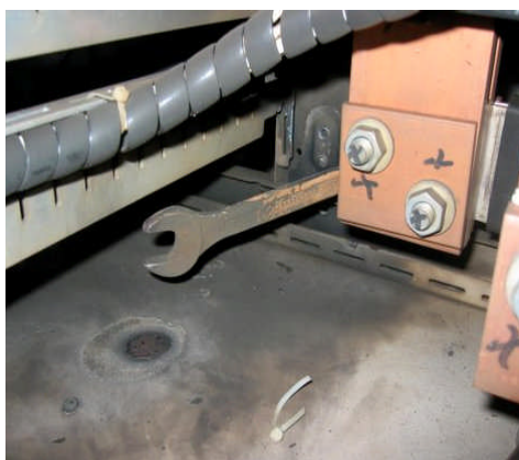
Short circuit in a power panel. Root cause was a forgotten tool. It was traced back to the manufacturer.
