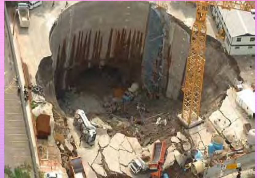
Day of collapse
