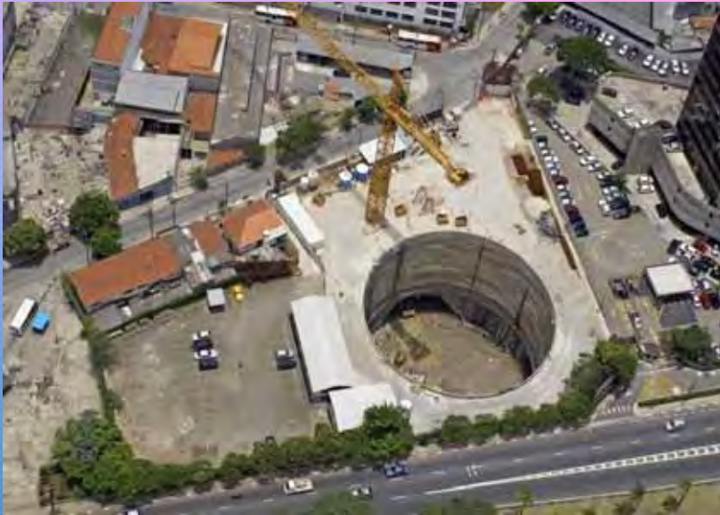
One week before collapse
