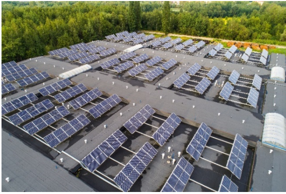
Air Gap provided (acceptable)
