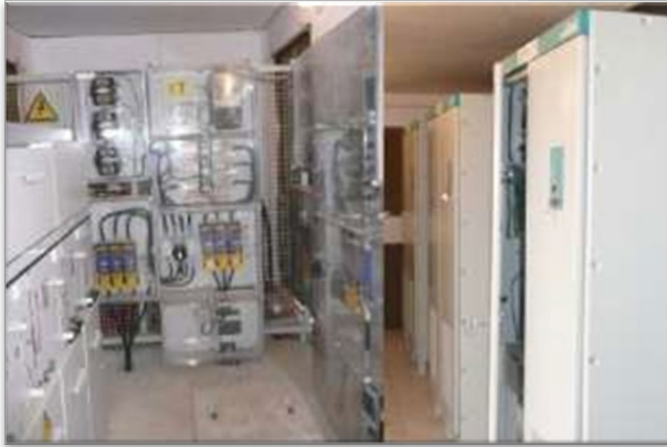
PV farm Substation
