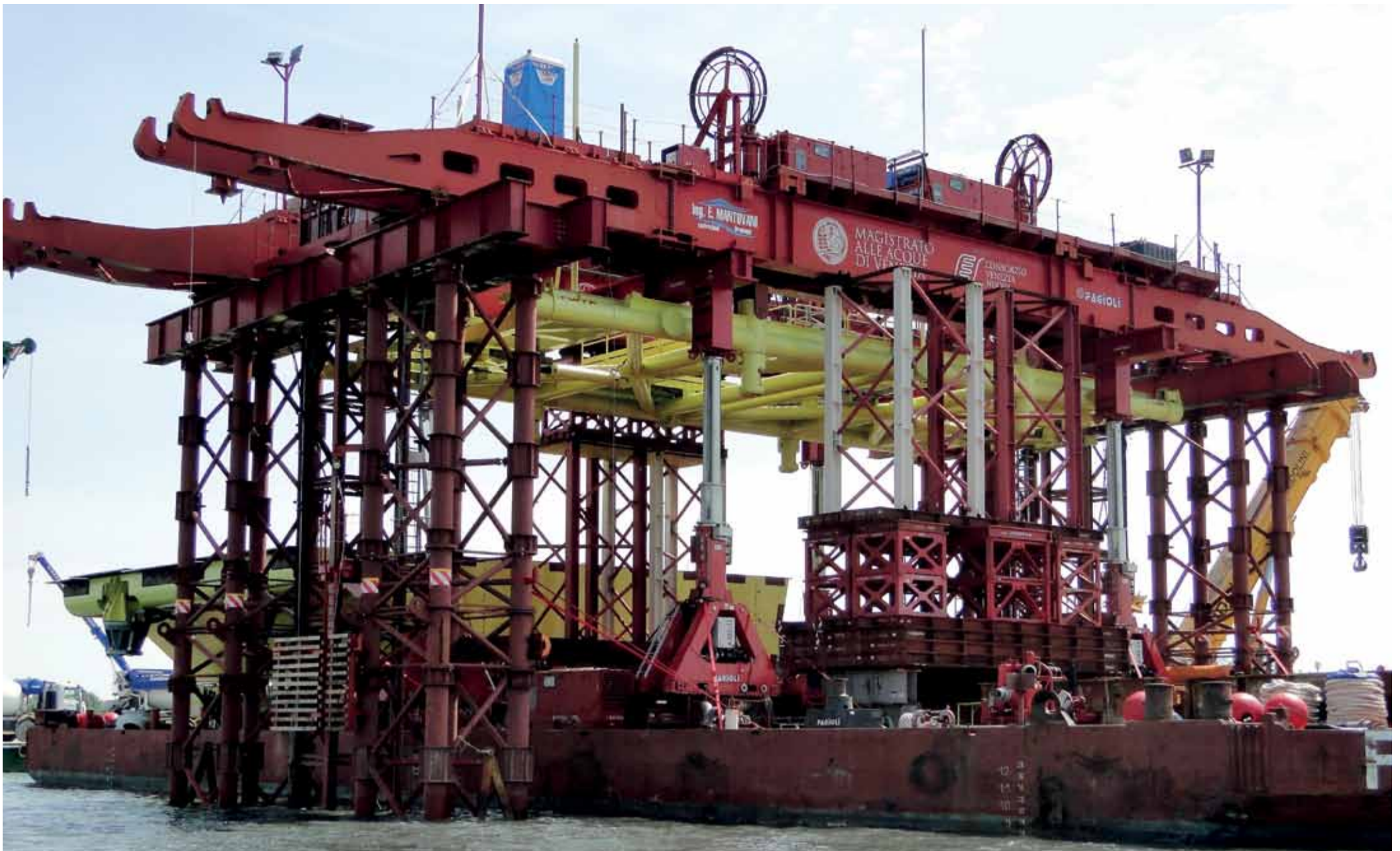
Special equipment for placing mobile sea barrier parts near Venice Silvano Bonelli | Munich Re Italy
