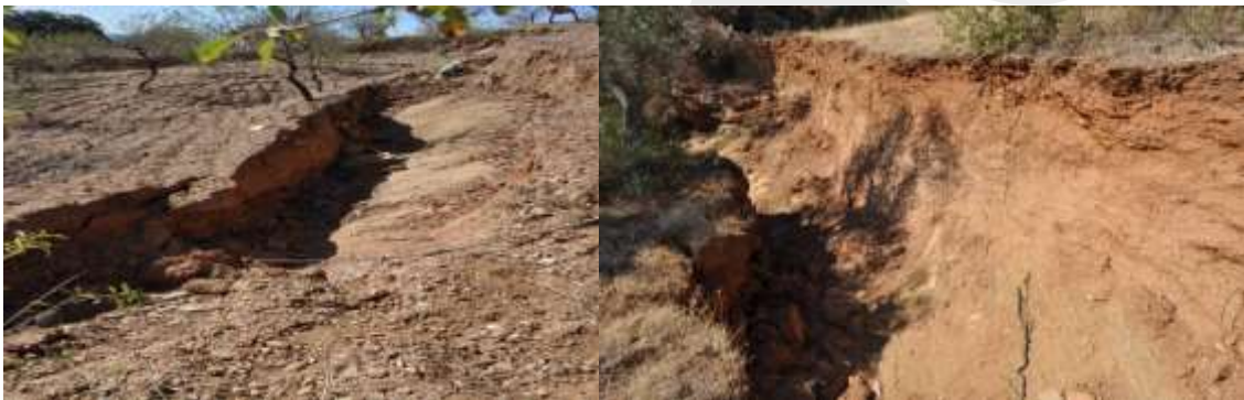
Photos 1&2: Views of the slipped area
