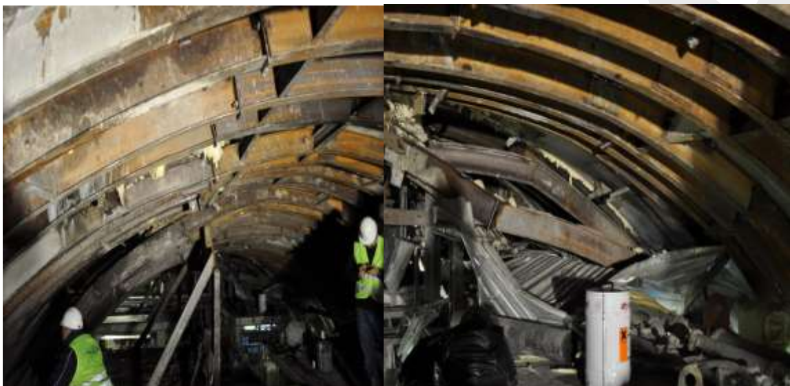
Photos 2 & 3: Partial collapse of the tunnel benches amongst stiff support resulting to the squeezing and damaging of the TBM
