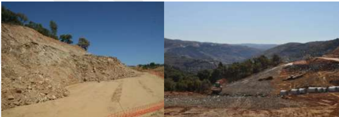
Photos 3 & 4: (a) earth mass fell on the already completed sub base of the motorway under construction, (b) works for re-routing the affected stretch of the motorway.
