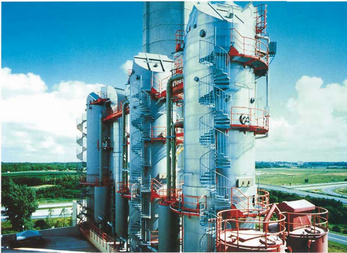
Flue-gas scrubbing towers in an MWT plant with three treatment lines
