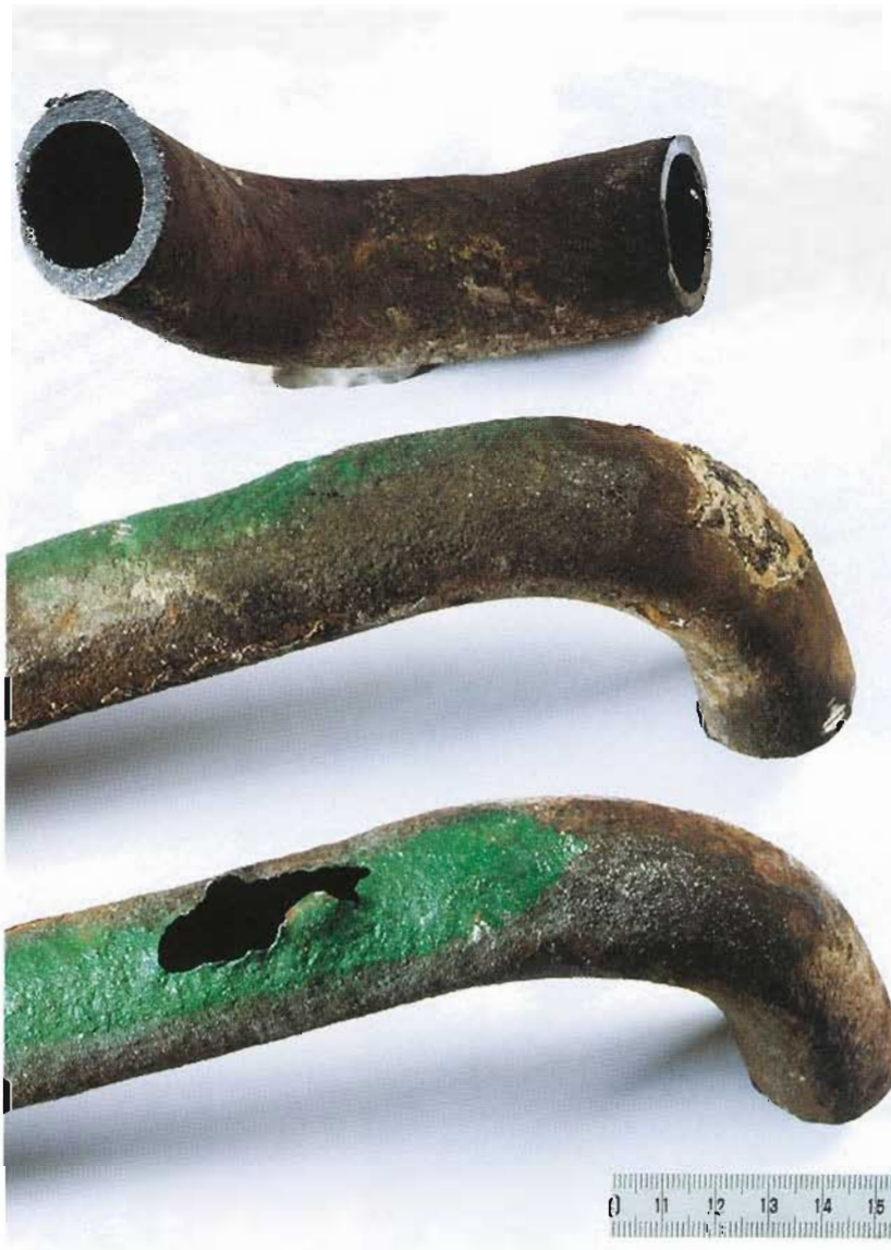
Corroded tubes from a boiler's superheaters. These tubes, which are not protected by refractory brickwork, are extremely exposed to corrosive and abrasive combustion gases.
