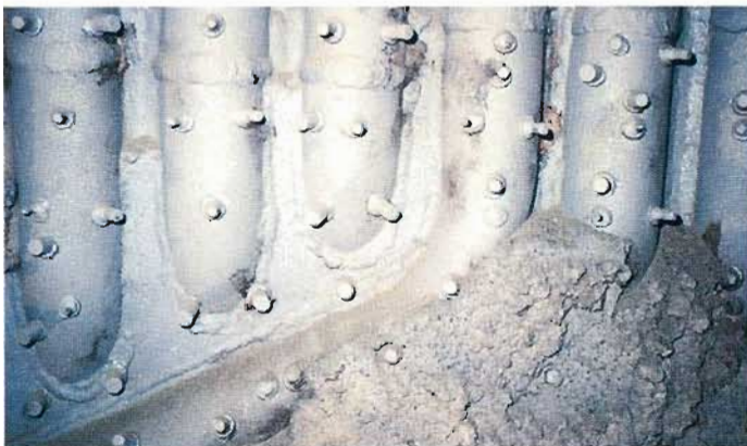
Damaged refractory brickwork (shot concrete) on the walls of the combustion chamber, made up of boiler tubes.
