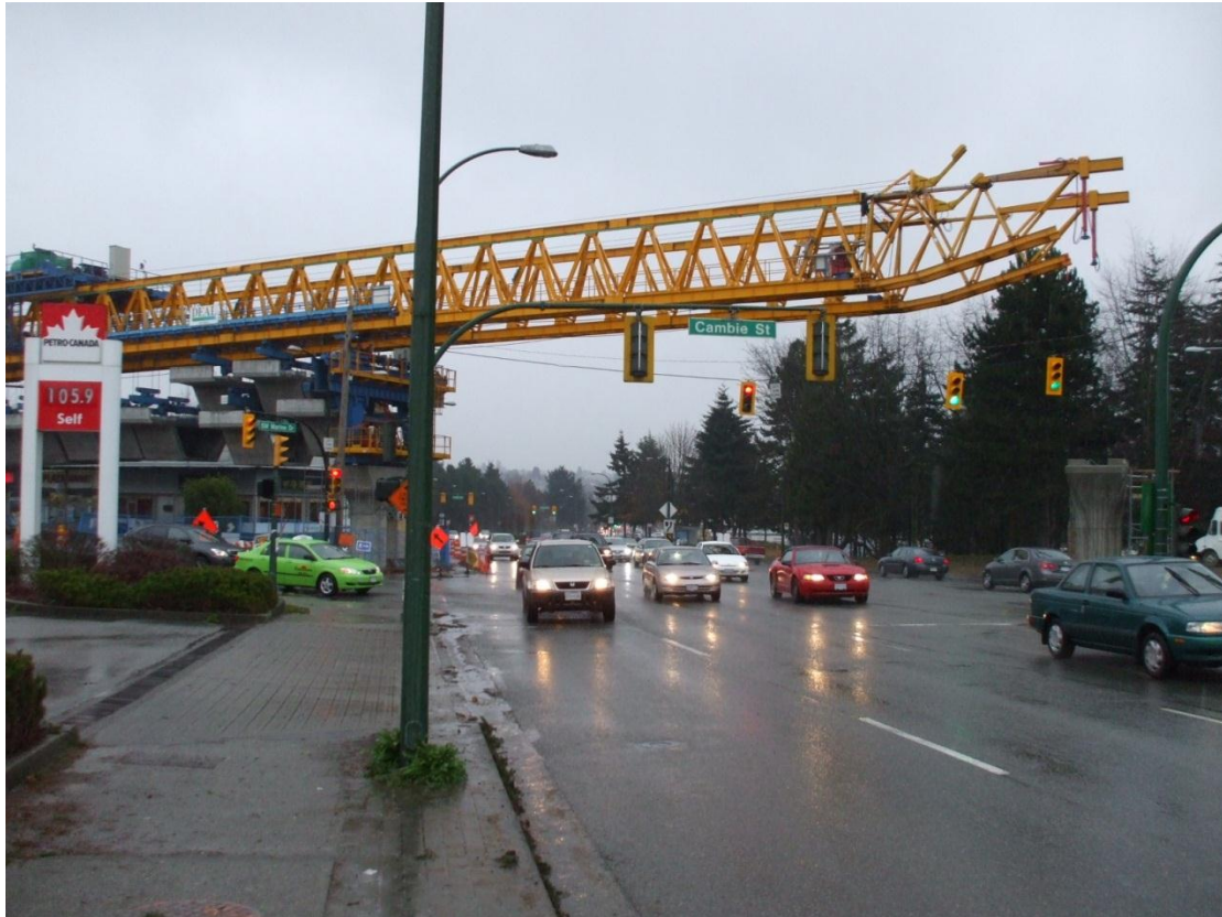
Erection gantry for elevated guideway segments – Vancouver – working directly above a live highway creates significant liability risks
