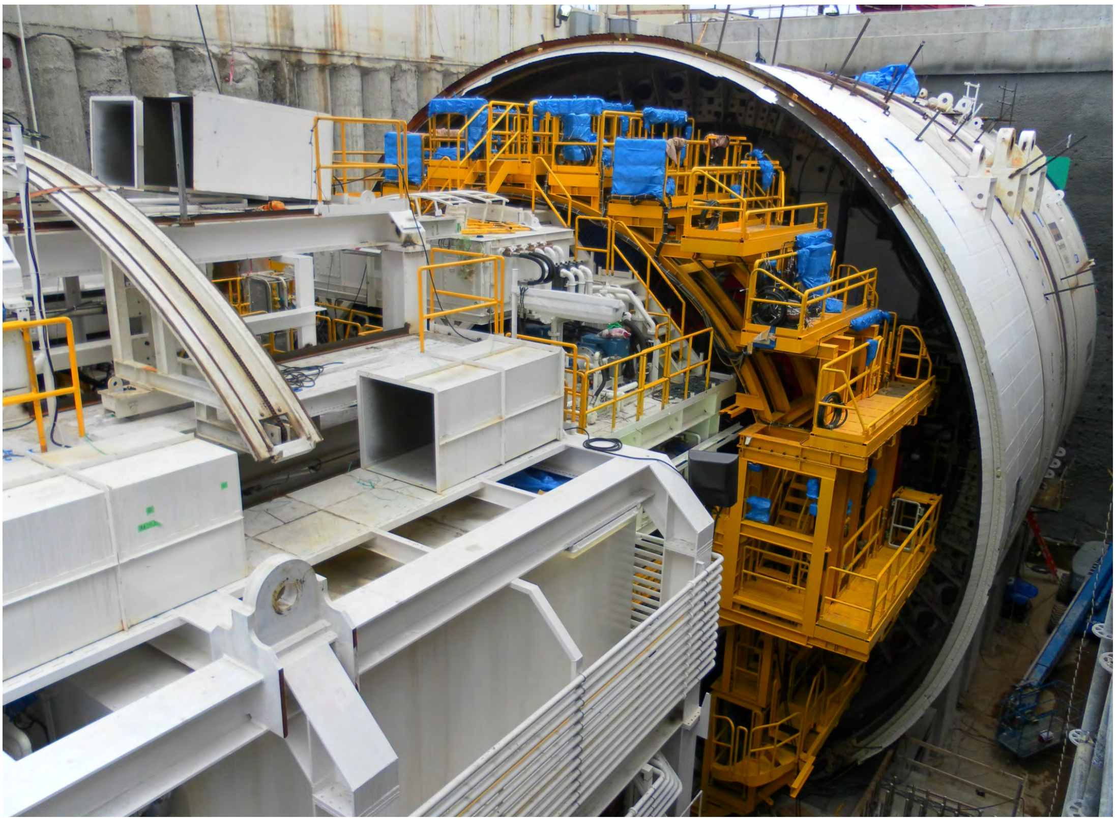
16 m diameter Tunnel boring machine at Seattle Alaskan Way Viaduct (Heiko Wannick, Munich Re)
