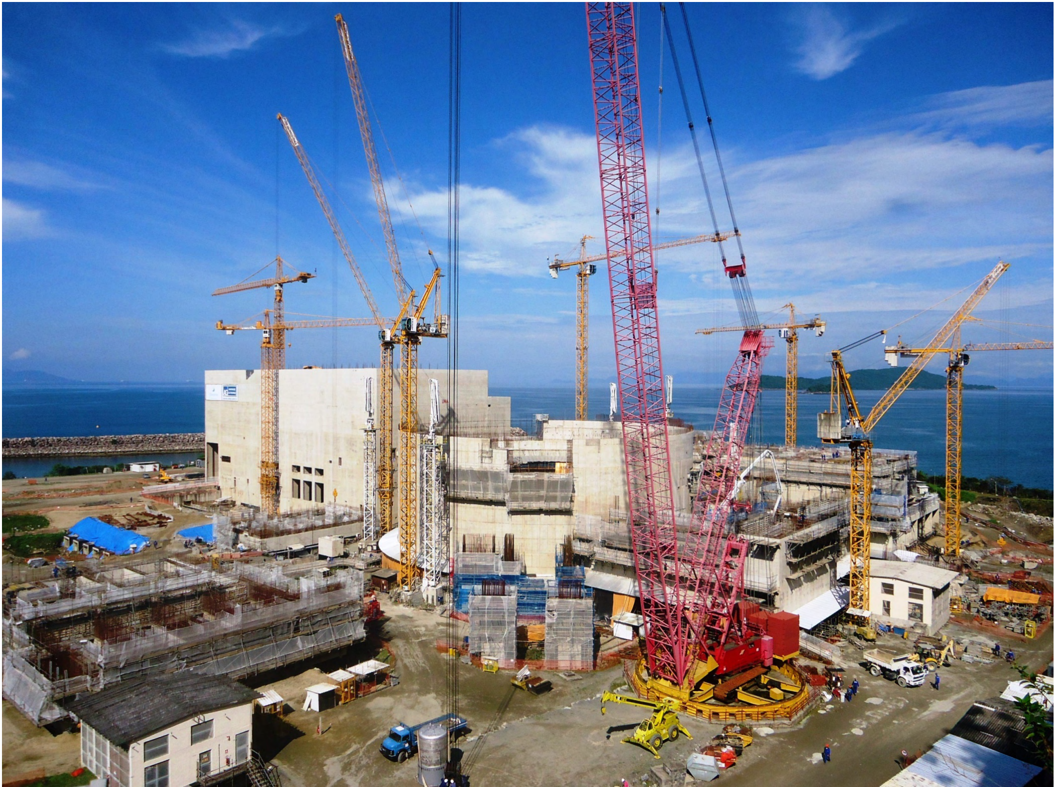
Civil Works Nuclear Power Plant Angra 3 Brazil – by Marco Barros, Allianz Brazil
