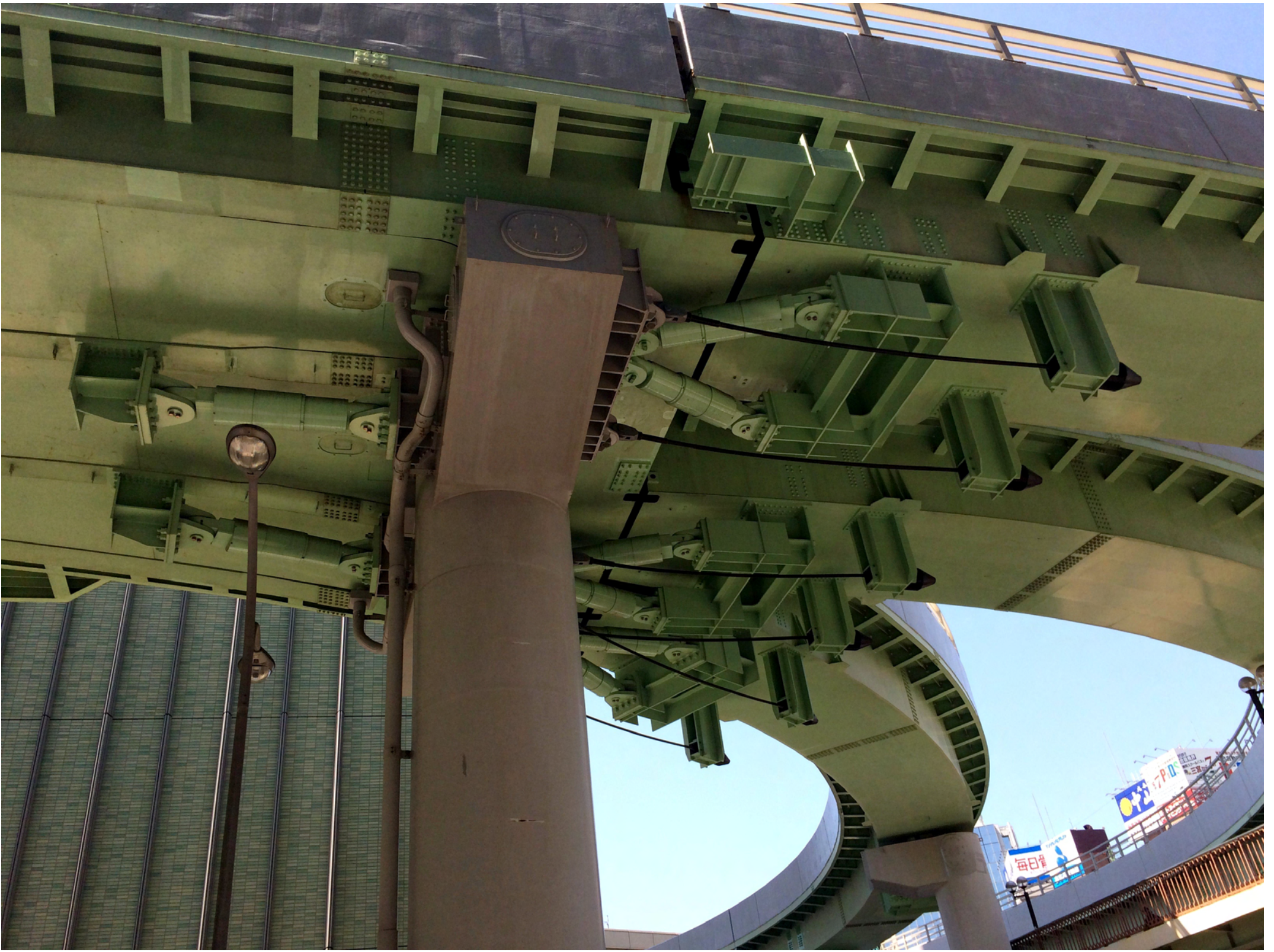
Railway bridge , Kobe (with EQ safety cables and shock absorbers) 2016 – Jürg Planta, Endurance
