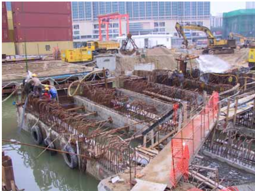
Tilted outfall structure
