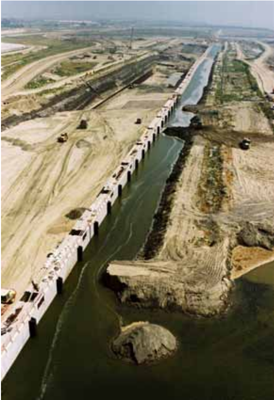
View of ditch and broken cofferdam
