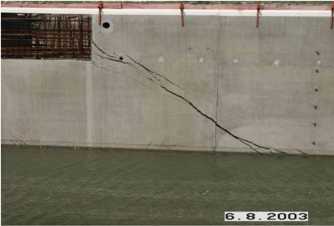
Cracks in the retention wall
