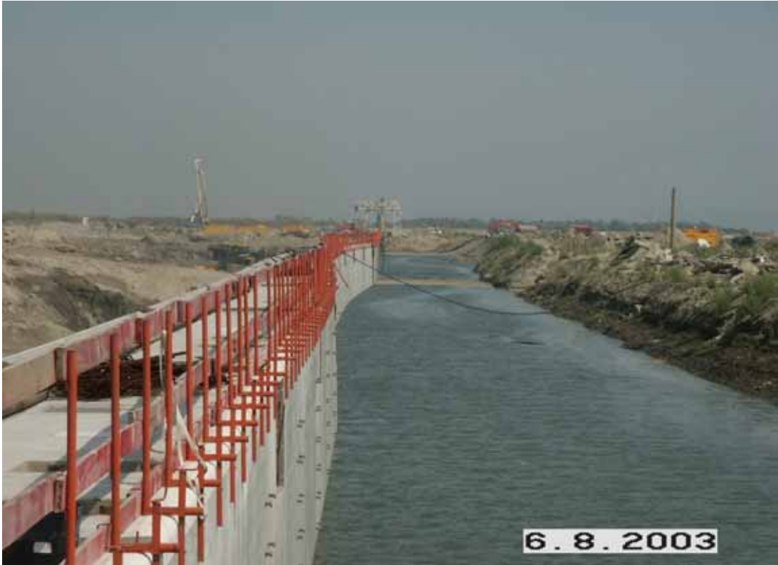
Deformed section of the retaining wall
