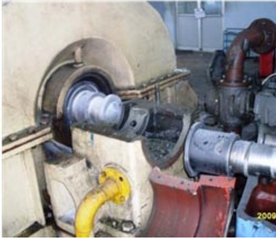
Turbine rotor shaft broken near journal
