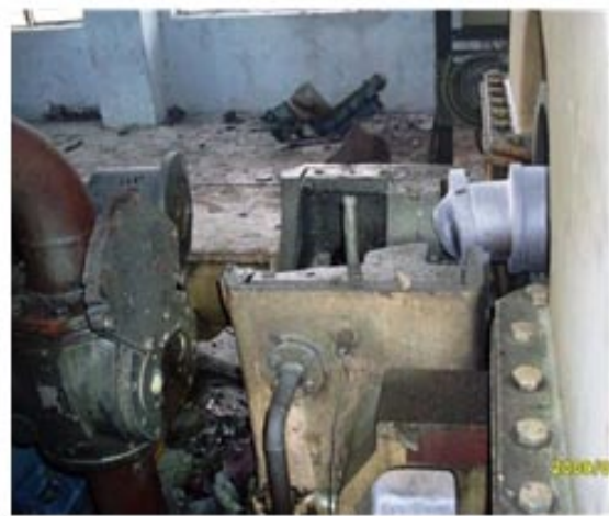
Rear bearing pedestal and coupling area
