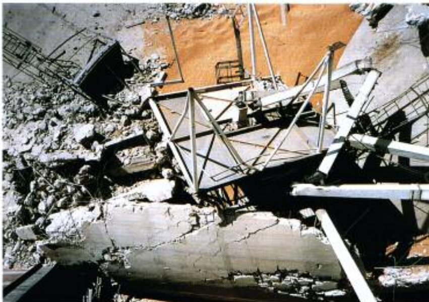
Debris of collapsed concrete grain silo
