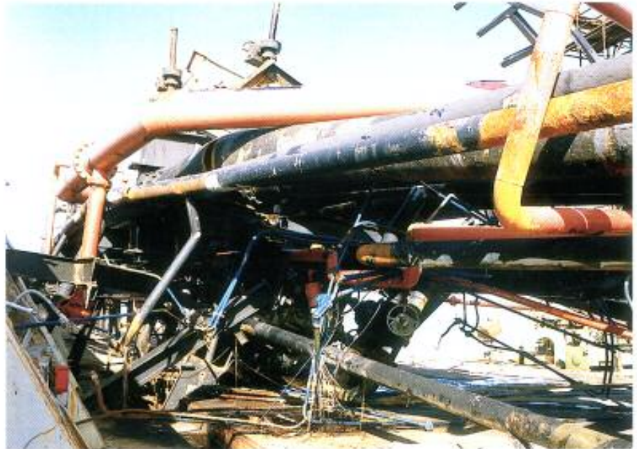
Fig. No. 225 Loading and unloading pipelines damaged beyond repair
