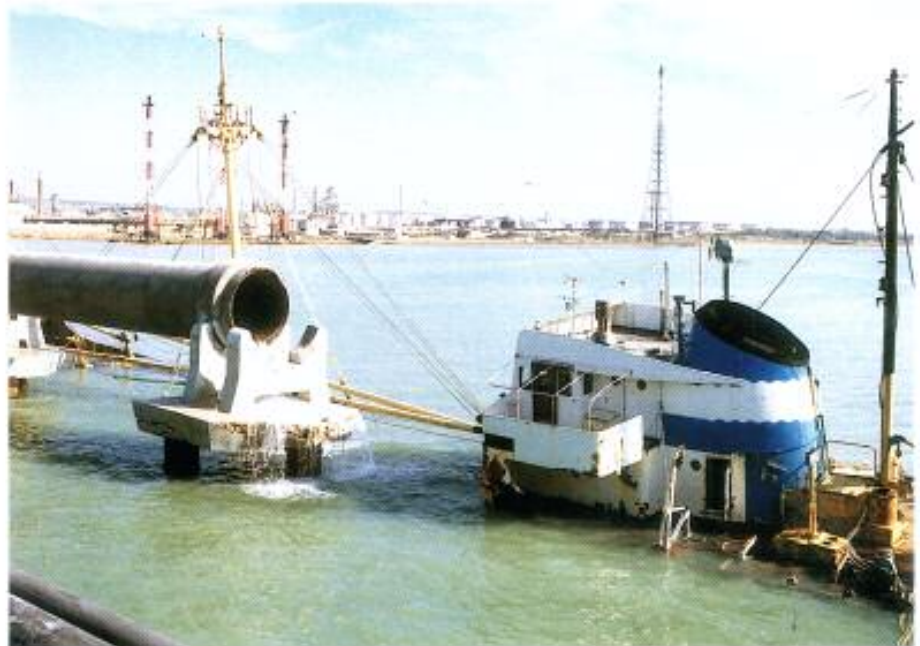
Fig. No. 226 Damage to pipelines and supports. One vessel sank to the seabed
