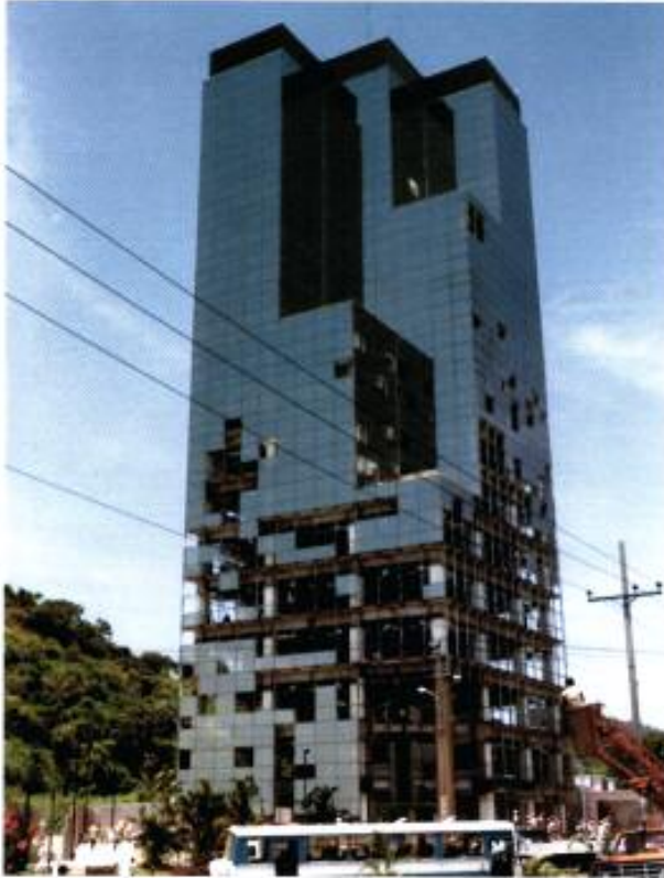
Damage caused by an explosion
