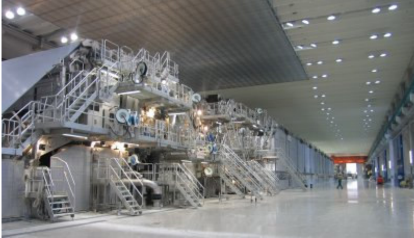
Figure 10, PM 12, Stora Enso, Kvarnsveden /3/
