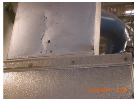
Figure 17: Wet corrosion of ash ducts
